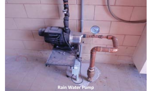
Rain Water Pump
